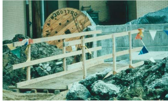
Walkways over excavations that are 6 feet or more in depth must be guarded to prevent falls.
