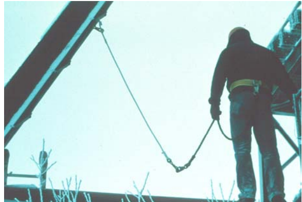
Unless approved by the manufacturer, snaphooks must not be attached to each other. Also, body belts are not used for personal fall arrest.
