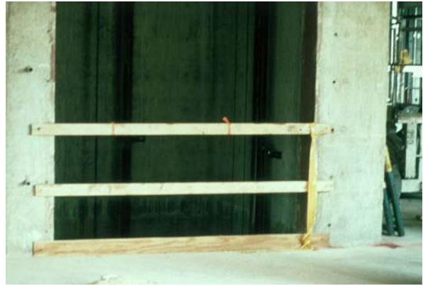
Elevator shafts and other similar wall openings must be protected against fall hazards.
