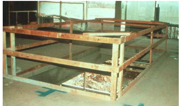
Wood guardrails must be made of at least 2"x4"s with spans not greater than 8 feet on center.
