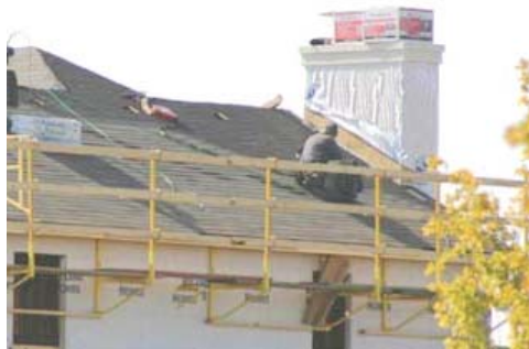
Figure 10 - An exterior bracket scaffold with guardrails being used to protect workers while weatherproofing.
