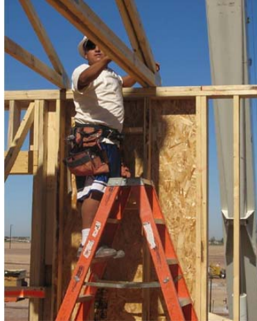
Figure 3 - Platform ladders can be set up inside a structure and used to install roof trusses.
